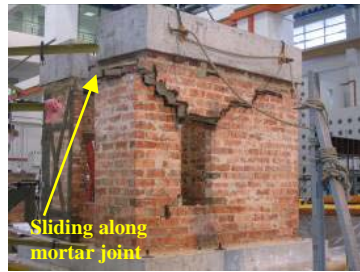
(b) PGA = 0.35 g: Upper portion of wall gave way
