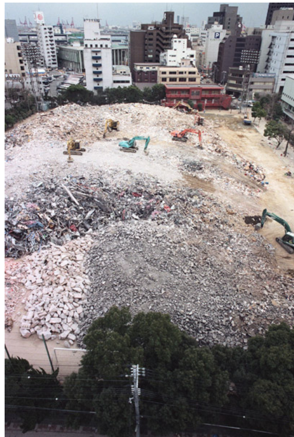
Photo 1: Accumulated disaster waste in a park in the central area of Kobe
